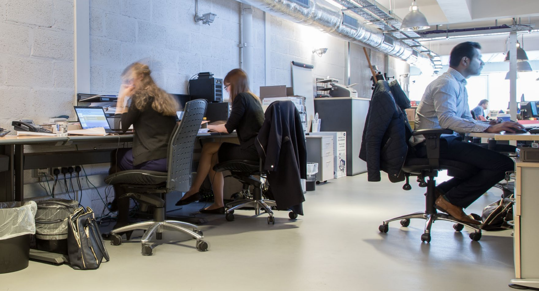
The existing substrate was planed and repaired prior to a pumped cementitious screed being laid to create a stable and level surface for the floor finish to be applied to.
